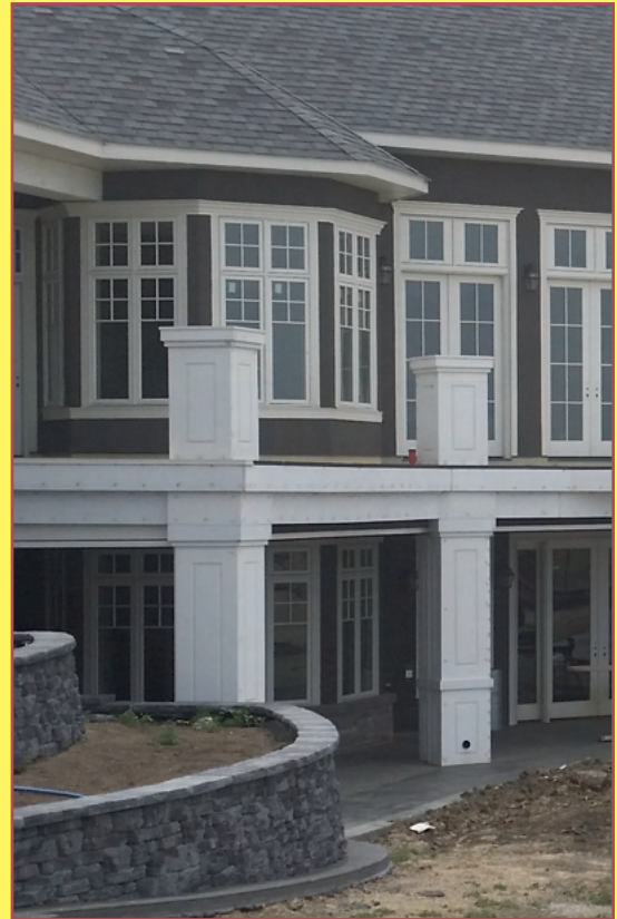
Photo above shows Spectis custom box column on a new home under construction
